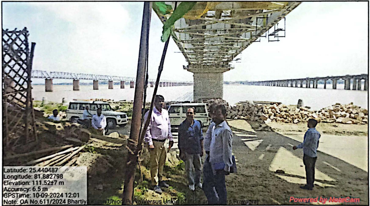
Photographs showing newly constructed Rail bridge over River Ganga near pier no. 25, towards Daraganj, Prayagraj on dt. 10.09.2024.
